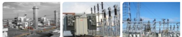
Electric Power Station & Transformers
